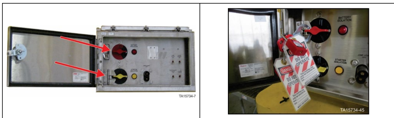
Figure 49. GEN 2 Battery Isolation Box – Battery isolation switch in OFF position with locks in place
