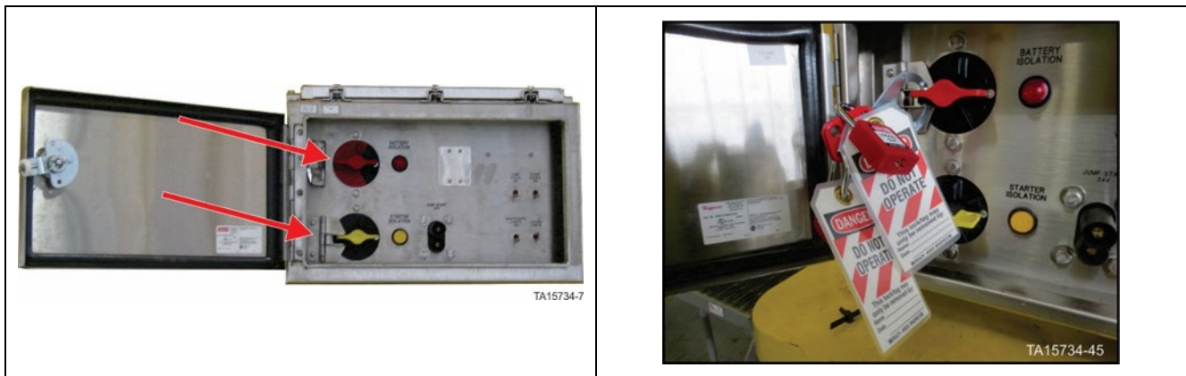
Figure 45. GEN 2 Battery Isolation Box – Battery isolation switch in OFF position with locks in place
