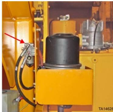
Location of compressor governor
