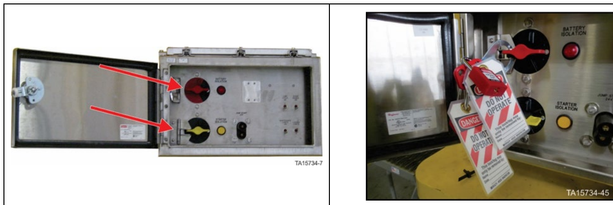
Figure 34. Battery Isolation Box – Battery isolation switch in OFF position with locks in place
