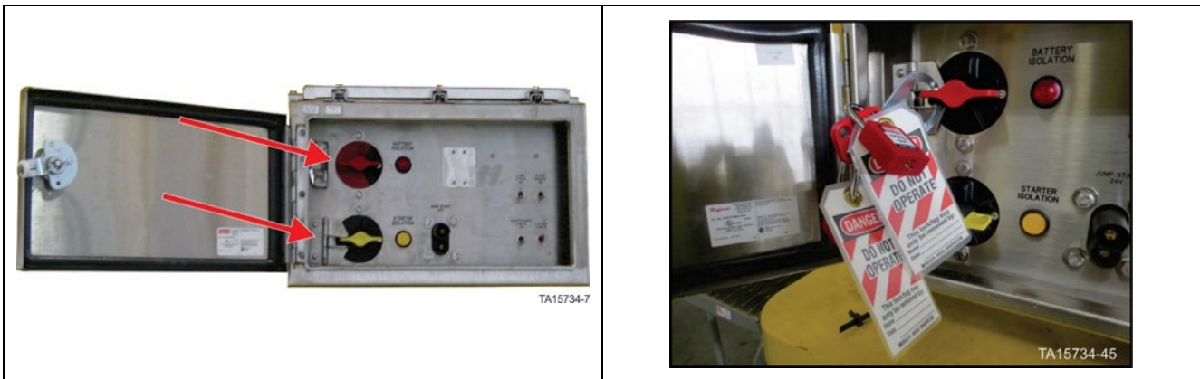
Figure 39. GEN 2 Battery Isolation Box – Battery isolation switch in OFF position with locks in place
