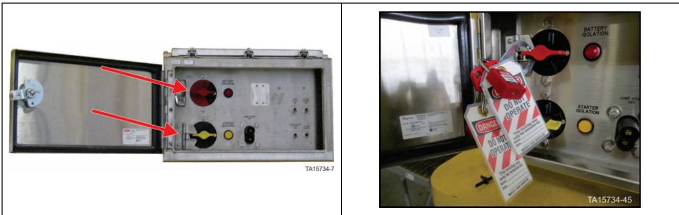
Figure 20. GEN 2 Battery Isolation Box – Battery isolation switch in OFF position with locks in place
